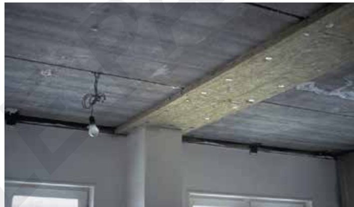
1.19 Protection of the bottom flange of an integrated beam with mineral wool boards. With a minimum plate thickness often a fire resistance of 120 minutes can be achieved.
